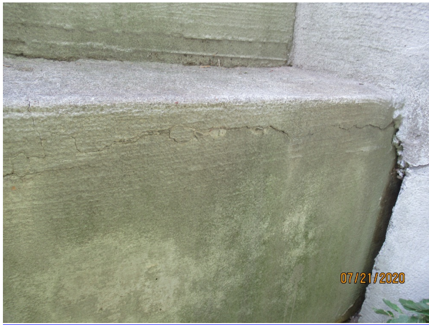
CRACK - BEAM "A", LT FACE AT ABUTMENT #1
