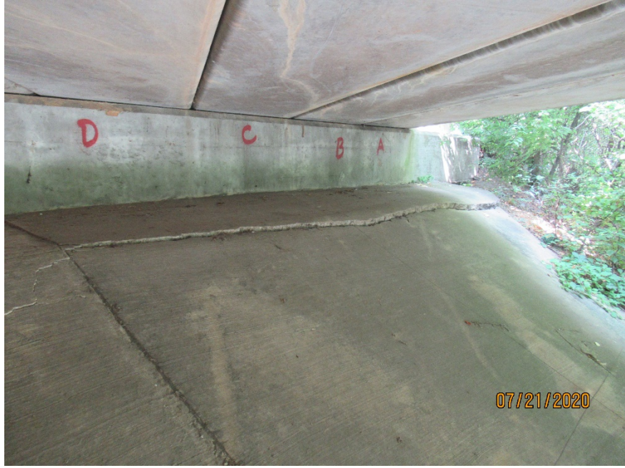
CRACK/SETTLEMENT IN SLOPE PAVEMENT - #1, LT
