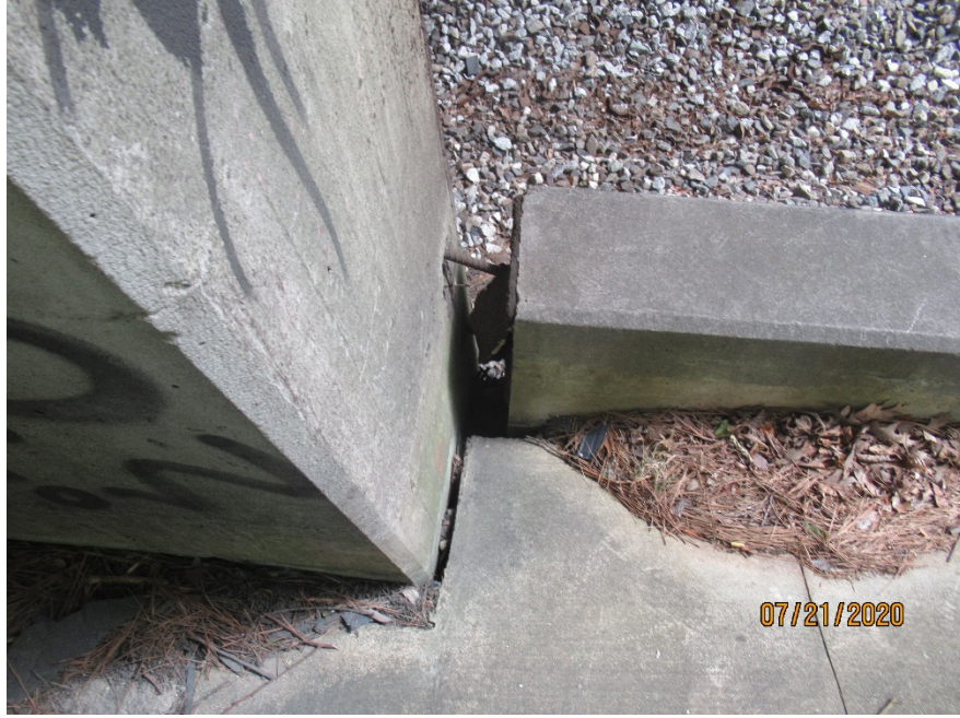
SEPARATION OF RETAINING WALL - BENT #1, RT
