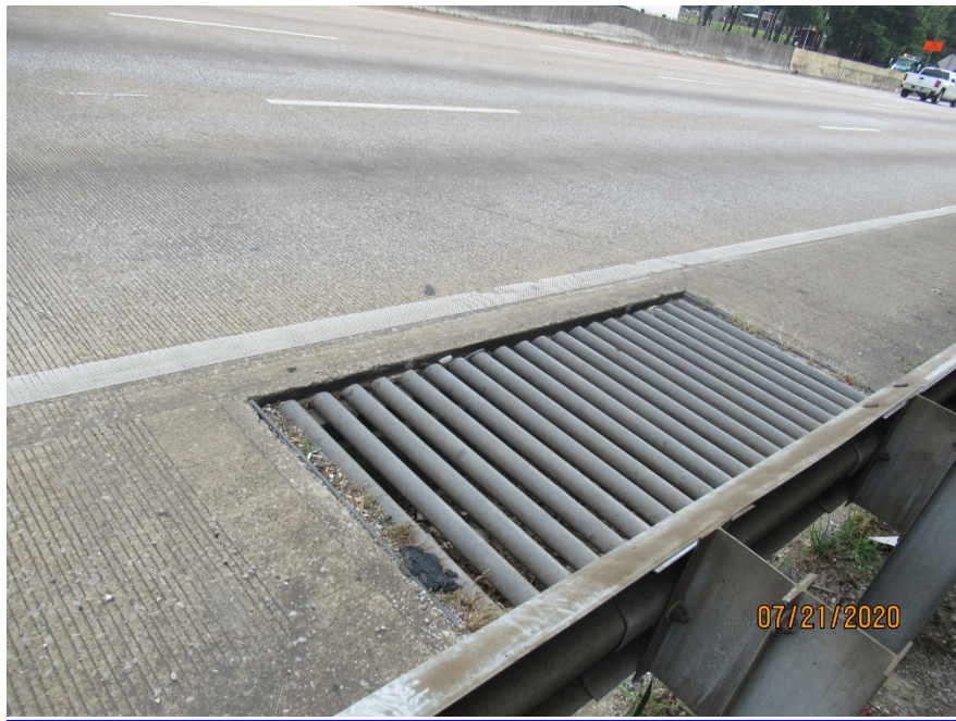
APPROACH DRAIN #1, RT - TYPICAL
