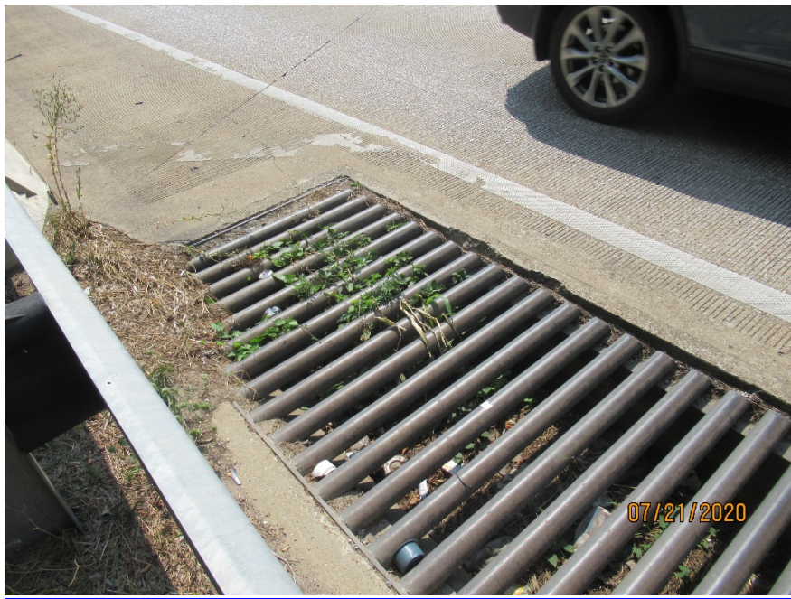
DRAIN CLOGGED - APPROACH #1, LT
