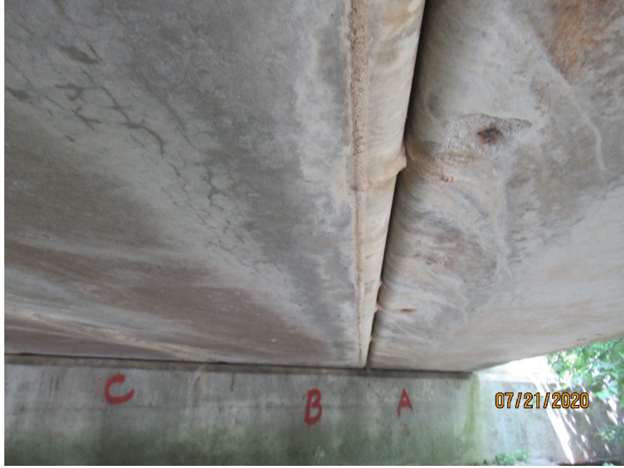
EFFLORESCENCE ACCUMULATION BETWEEN BEAMS "A" AND "B" – SPAN #1
