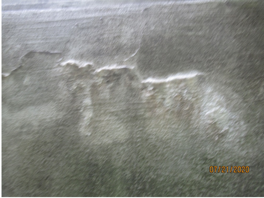
CRACK W/ EFFLORESCENCE - BEAM "A", LT FACE AT ABUTMENT #1
